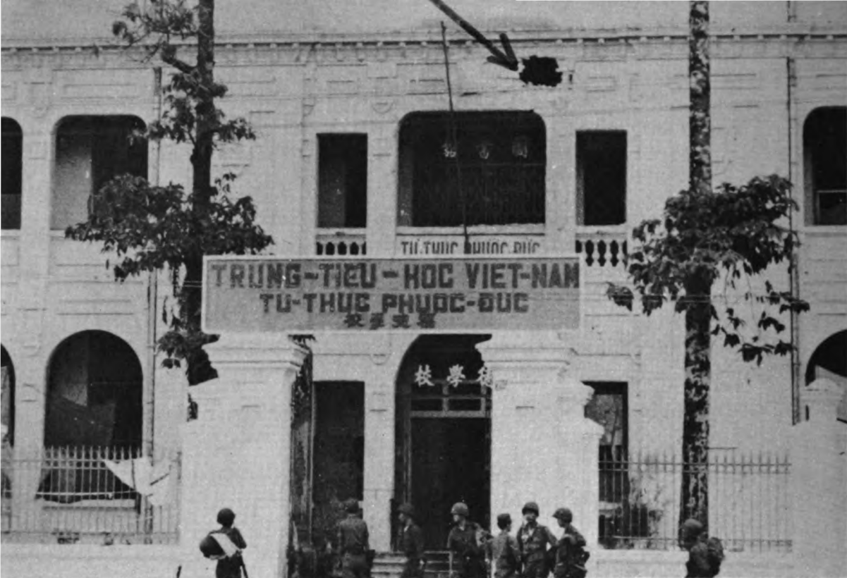
Hole opened in a wall of Phuoc Duc Private High School by a rocket launched by mistake from an armed helicopter.
