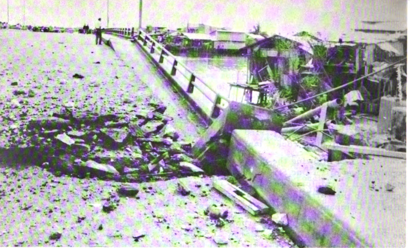
In the early hours of 5 May 1968, the Phan Thanh Gian bridge was blown up by VC agents. Some damage was reported as may be seen on this picture.
