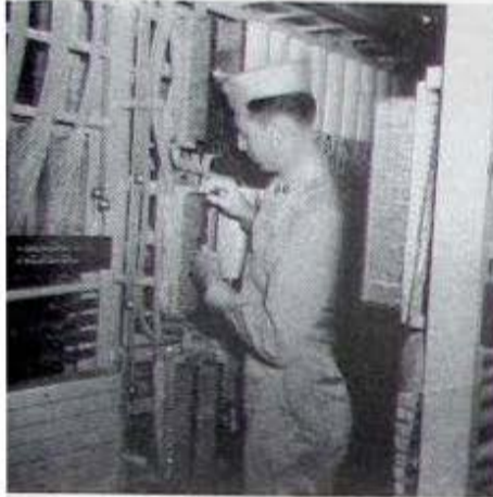
Base signal telephone frames, 18 CS
